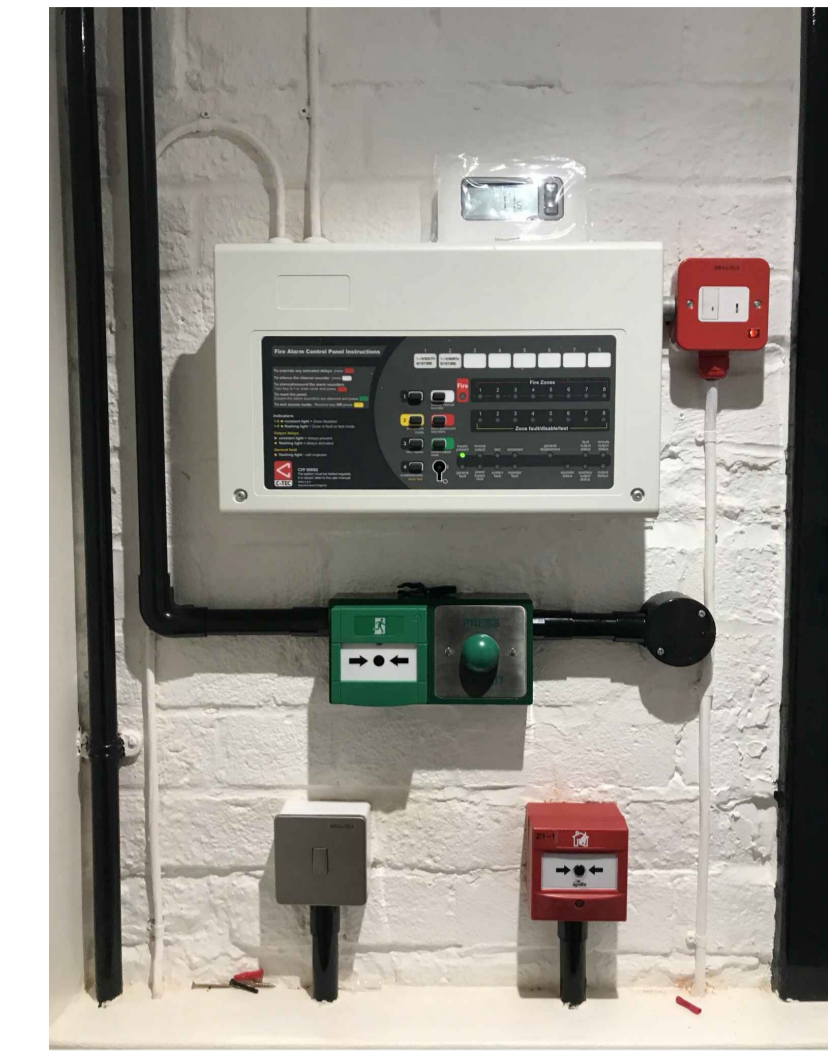
2 GROUND FLOOR FIRE ALARM PANEL (FAP)
